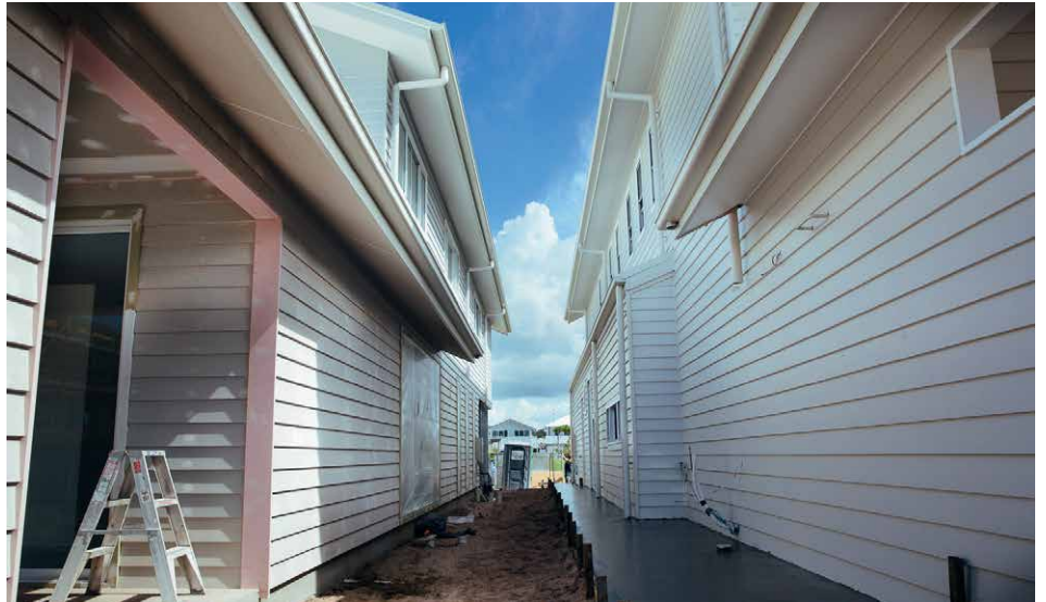
Above: Homes under construction, various stages of painting, ready for top coat.
