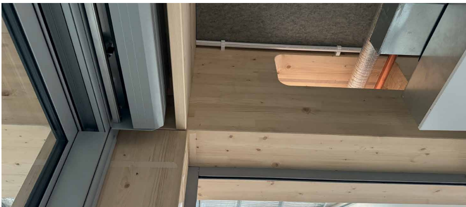
Above: The prototype at Allied Mass Timber site is used for training many different trades.
