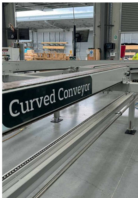
Above: The unique curved conveyor allows the stud and noggins to travel to the auto framer.
