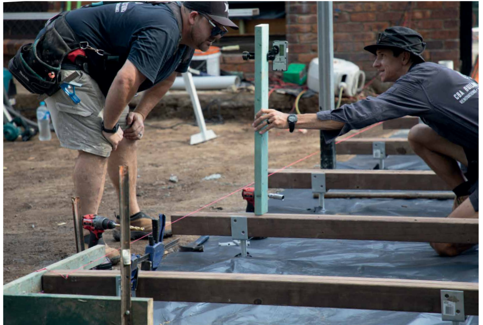
Above: Decks should always be considered as a whole system. Here, steel stirrups sunk into concrete help to ensure good drying periods for the timber above, regardless of how wet the summer is.
