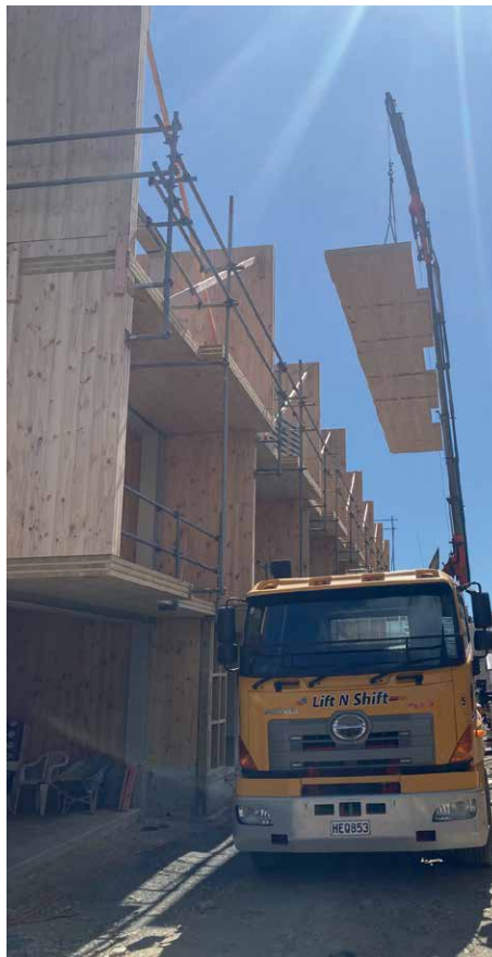
Above: Hardy St, Nelson. There’s a growing recognition of mass timber’s role in reducing the construction industry’s carbon footprint.
