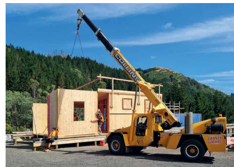
Above: Once delivered onsite, a modular home's connections are completed in four weeks.
