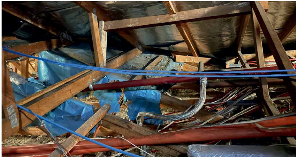
Above: This tangle of services in the roof of an aged care home adds load that needs specific designs.
