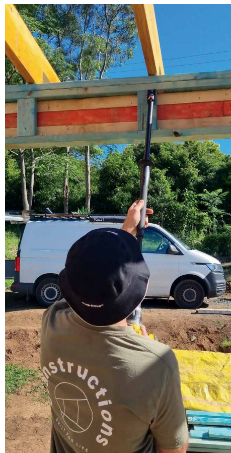
Above: Installing Simpson truss screws using a Quik Stik, eliminating the need to work at height.
